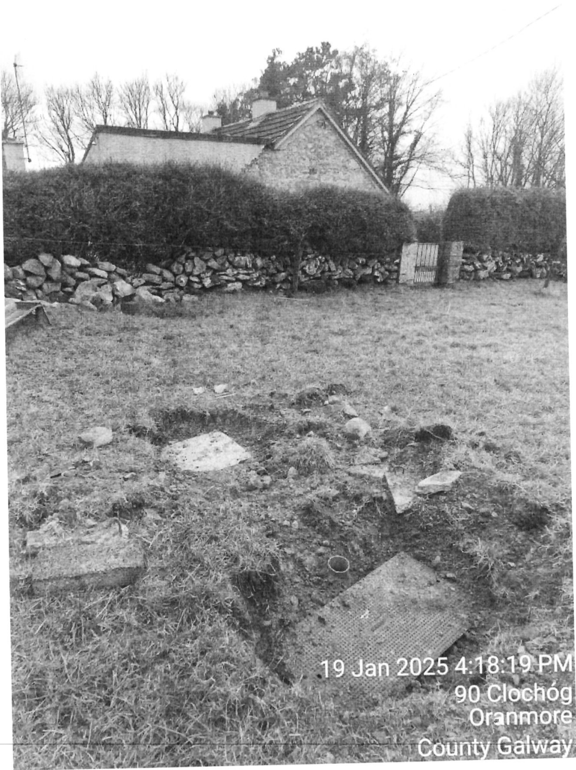
Fig 04. Photograph of exposed septic tank – location as per drawings
