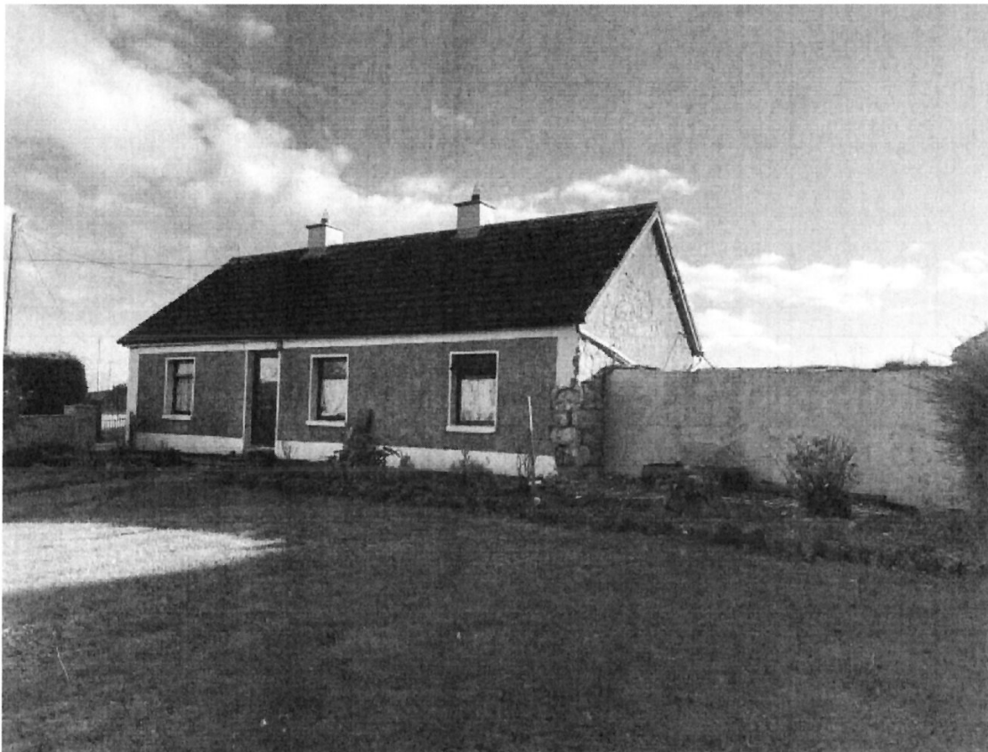
Fig 01. Front of cottage. – prior to remediation works to external render finish.
