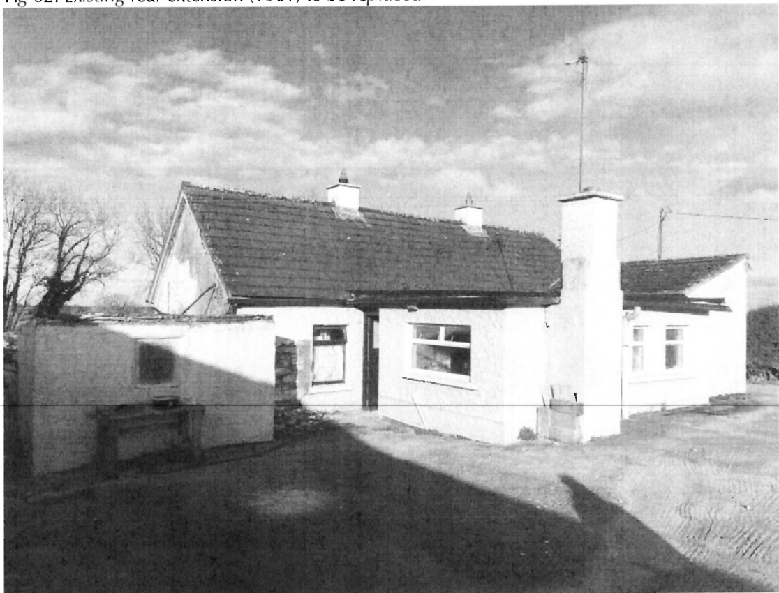
Fig 03. Existing rear extension (1961) to be replaced – footprint of proposed extension to be broadly consistent with existing.
